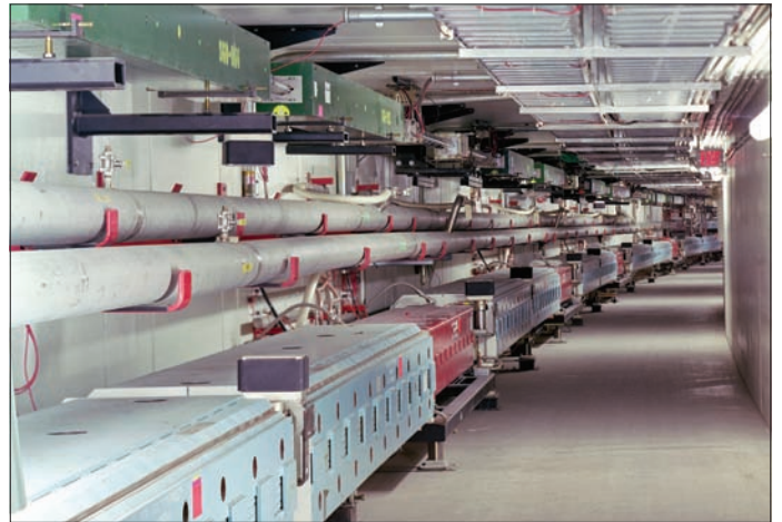
The Main Injector ring, below, with the green magnets of the Recycler suspended from the ceiling. (Image credit: Fermilab Visual Media Services.)
