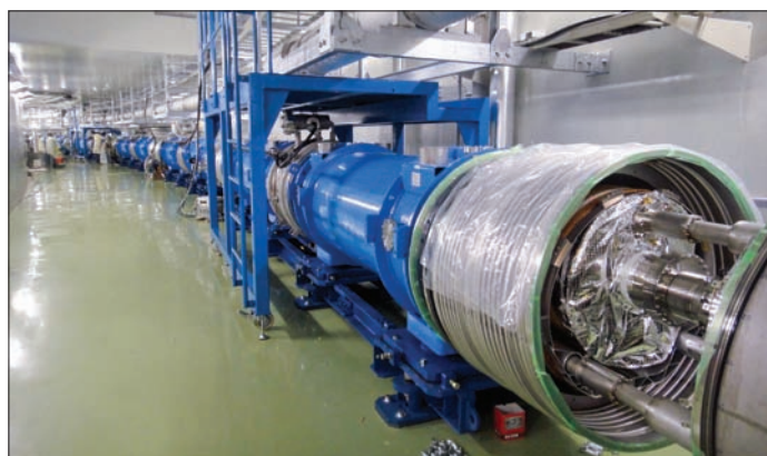
Fig. 3. J-PARC primary proton beam line and the superconducting combined-function magnet string.
