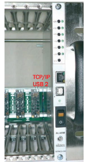
NIM control panel
